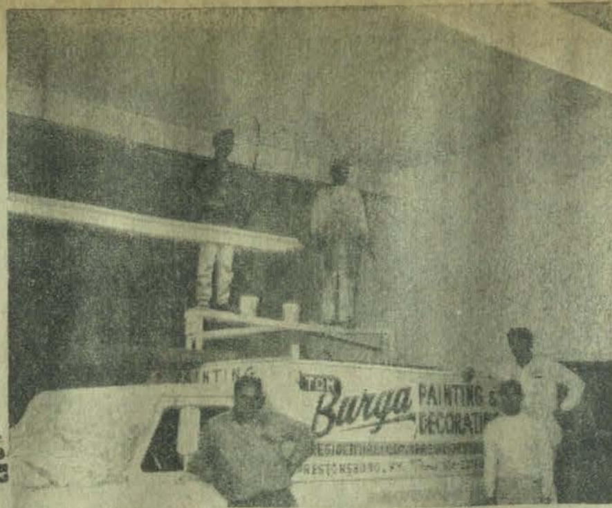
Tom Burga (left), painting contractor, with employees at work on interior of new plant building here. Mr. Burga gave his services to get the building ready for occupancy Dec. 1.
