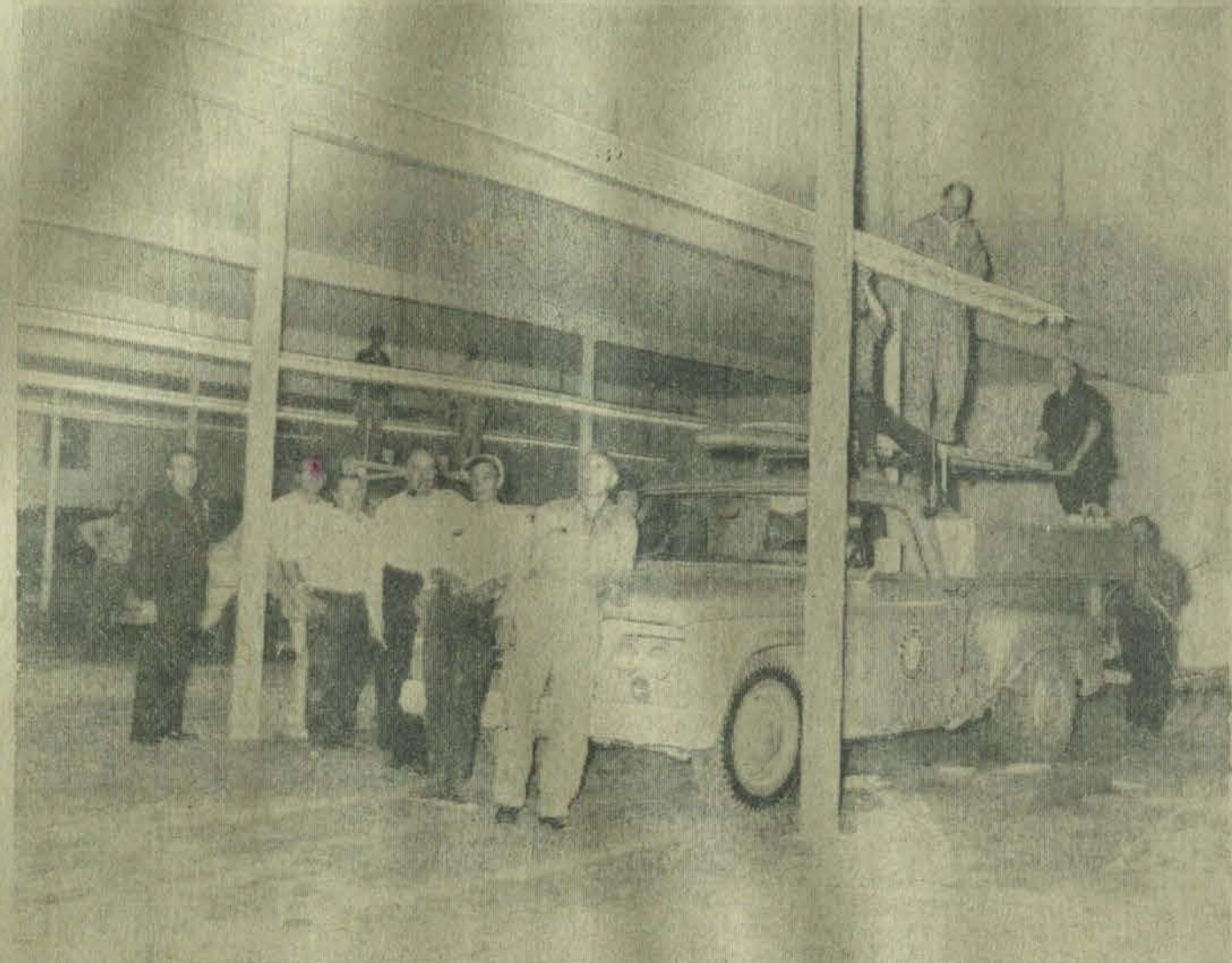
OLD-FASHIONED "WORKING" speeds building to completion for plant here. In foreground, from left—Marvin Music, Tom O. McGuire, Bill May, Russell May, James Stamper, Irvin Harris. Kentucky Power Company men are on truck, Herbert Kincaid, district manager, nearest wall. At left, in background, is Tom Burgz, who did the paint work. Others in photo were not identified.
