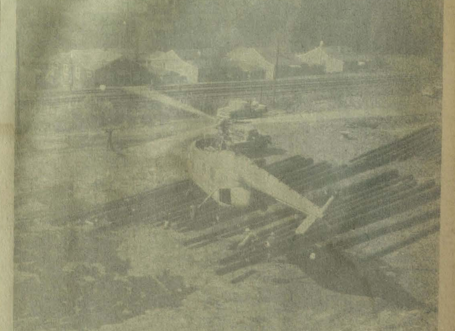
Helicopter hovers over power pole at Stone material center. Moments later, it was connected with pole and on way to where work crews stood by to receive its cargo.
