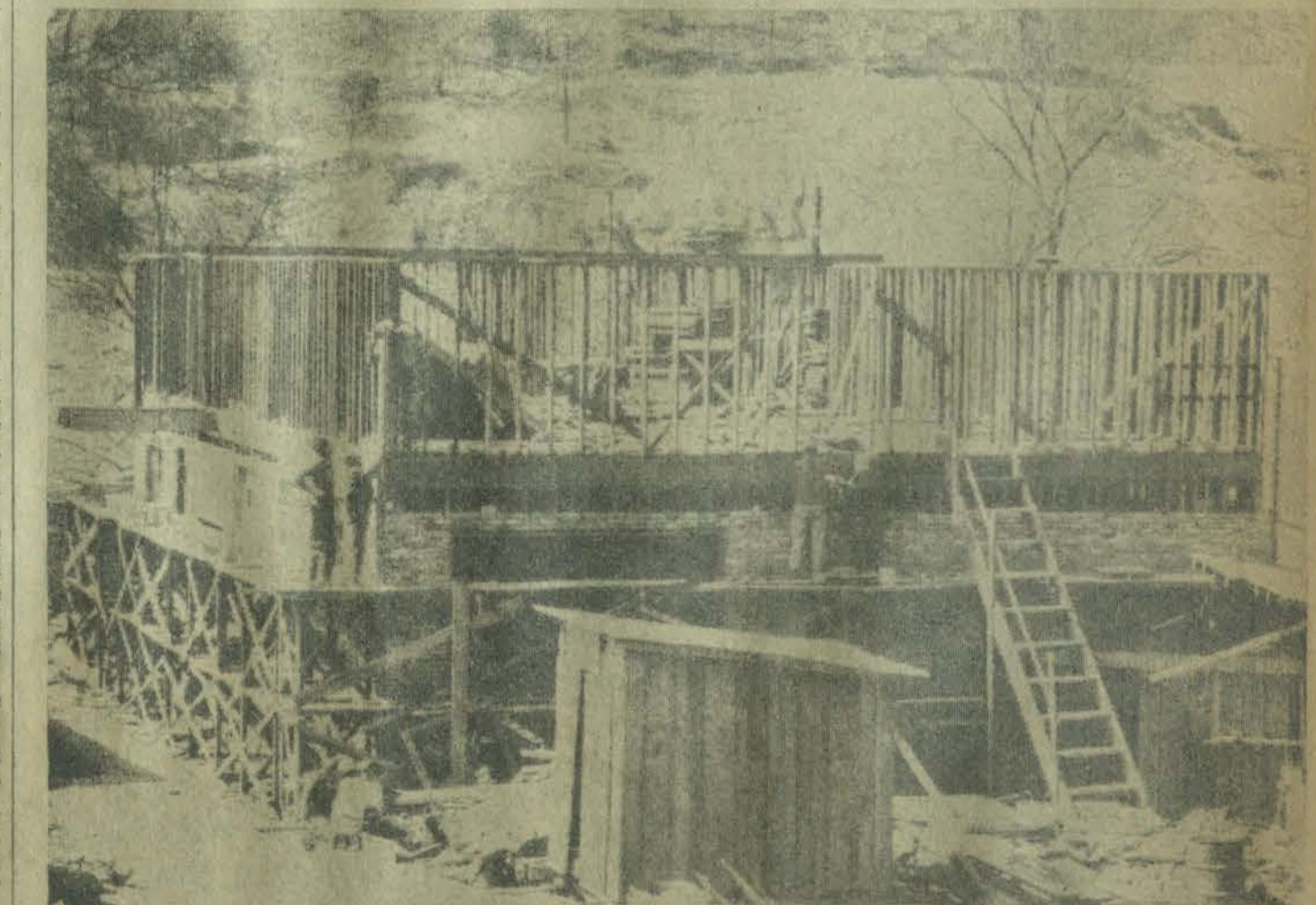
THE OLD BECOMING SOMETHING NEW. Workmen are shown building with bricks from the old Floyd county courthouse the first structure to be erected in Prestonsburg's recreation area, at the upper limits of West Prestonsburg. The two-story building under construction will house on the ground floor a garage and bulk concessions, plus storage space. On the second floor will be a five-room apartment and two three-room apartments for the park manager and other personnel.
