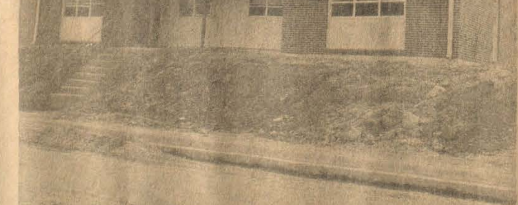
One duplex unit of the $655,000 low-rent public housing complex being constructed at the "Forks of Beaver," near Martin, is shown as the project nears completion. The housing facilities there are located on a hillside facing on Ky. 80 and overlooking the valley.
