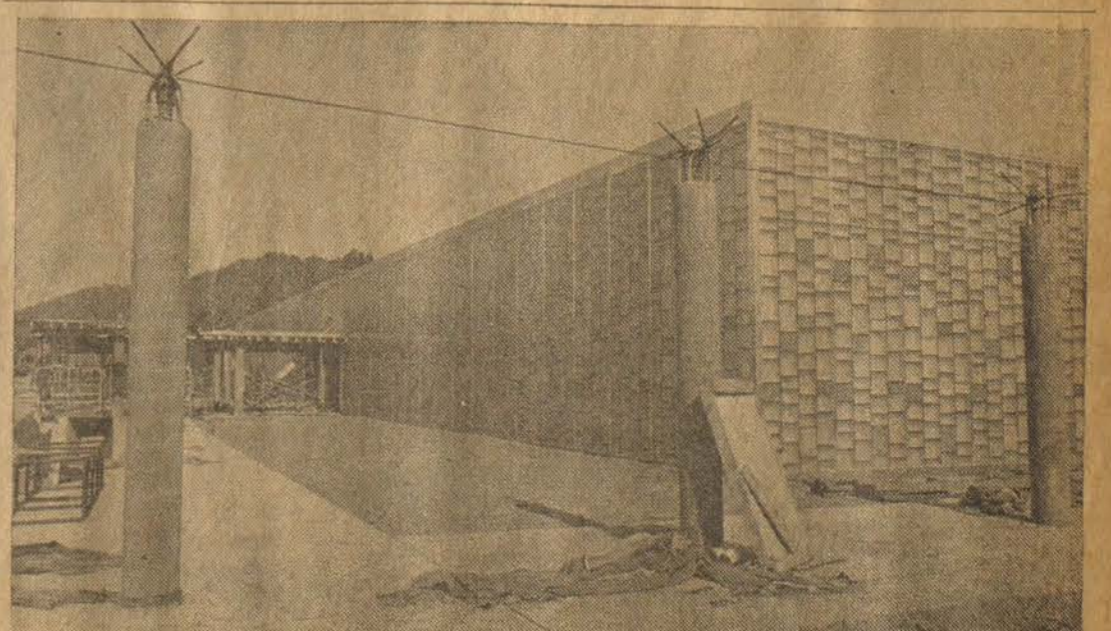
PRESTONSBURG COMMUNITY COLLEGE, scheduled to open this fall, takes form in these photos. The top picture shows the translucent fiberglass exterior of the air-conditioned, 35,000-square foot building. The $899,690 structure includes 20 classrooms, 14 offices, and a library and is located on a 40-acre site.
