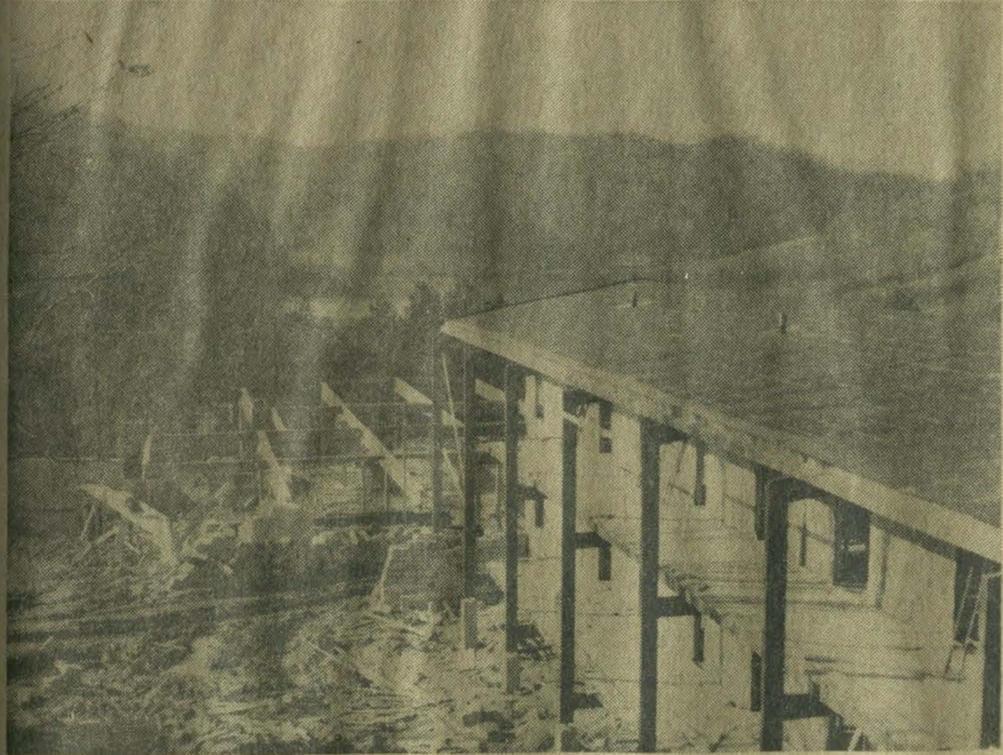
THIS VIEW OF DEWEY LAKE will be seen by guests at Jenny Wiley State Park lodge. Construction is over one-third complete on the new lodge at the park near here. At right is a portion of one of the three guest units, each containing 12 bedrooms. Each of the 36 rooms will have a private balcony overlooking the lake below. The steel girders in center background are the base for an unusual six-sided structure housing on the lower level a dining room seating 200. The hexagonal-shaped building will also house a lobby, park offices, gift shop and a large lounge which can be divided by sliding doors into four private meeting rooms.
