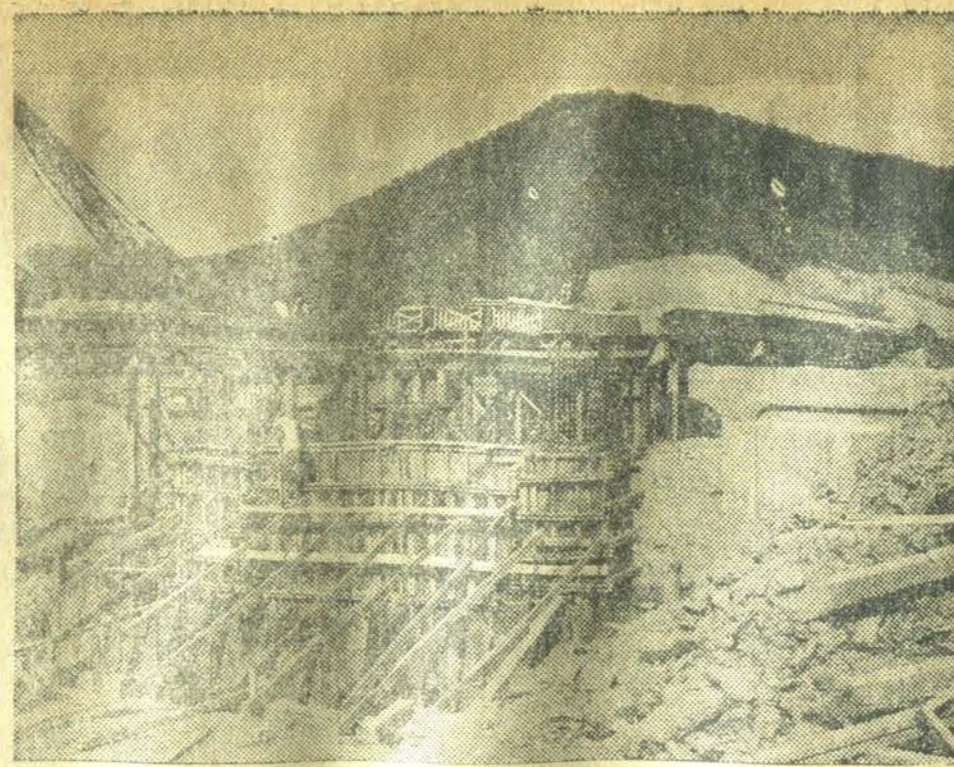
THIS BRIDGE, when completed, will be one of five to cross the Red River or its tributaries as the Eastern Kentucky Turnpike cuts its way from Winchester to Campton. This twin-span structure near Roslyn is the longest, measuring 460 feet in length.
