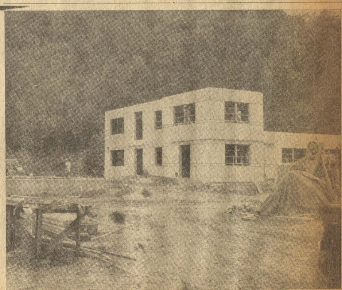
NEW WATER PLANT BUILDING in Mayo Addition to Prestonsburg, part of the big construction program which is expected by mid-December to see a new water system in operation here. The building is of steel-reinforced concrete and contains no wood, inside or out.
