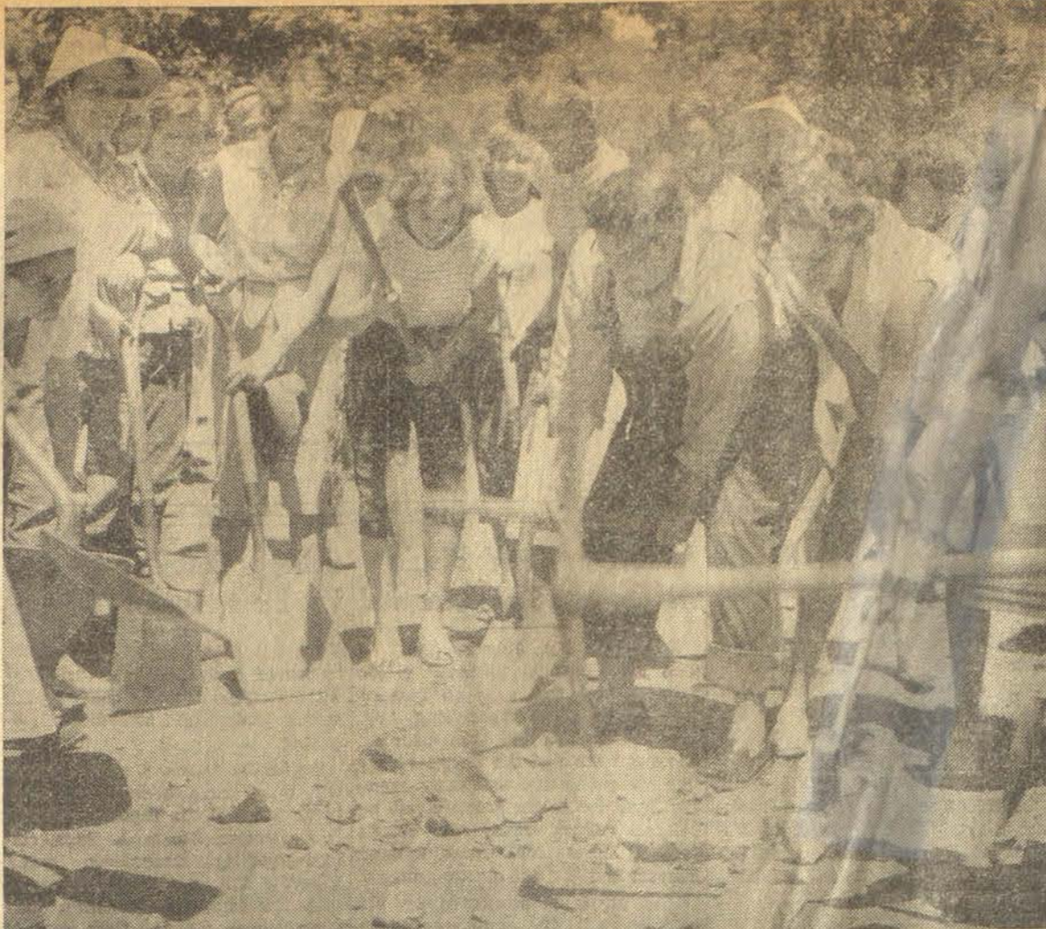
Auxiliary women turn out to work recently on the highway in protest to its neglect by the Highway Department. The aroused women, besides wielding pick and shovel on the road, turned to with hammer and nails to repair the bridge over Big Sandy there. Resumption of work on the road was promised by Rural Highway Commissioner J. B. Wells, Monday of this week.
