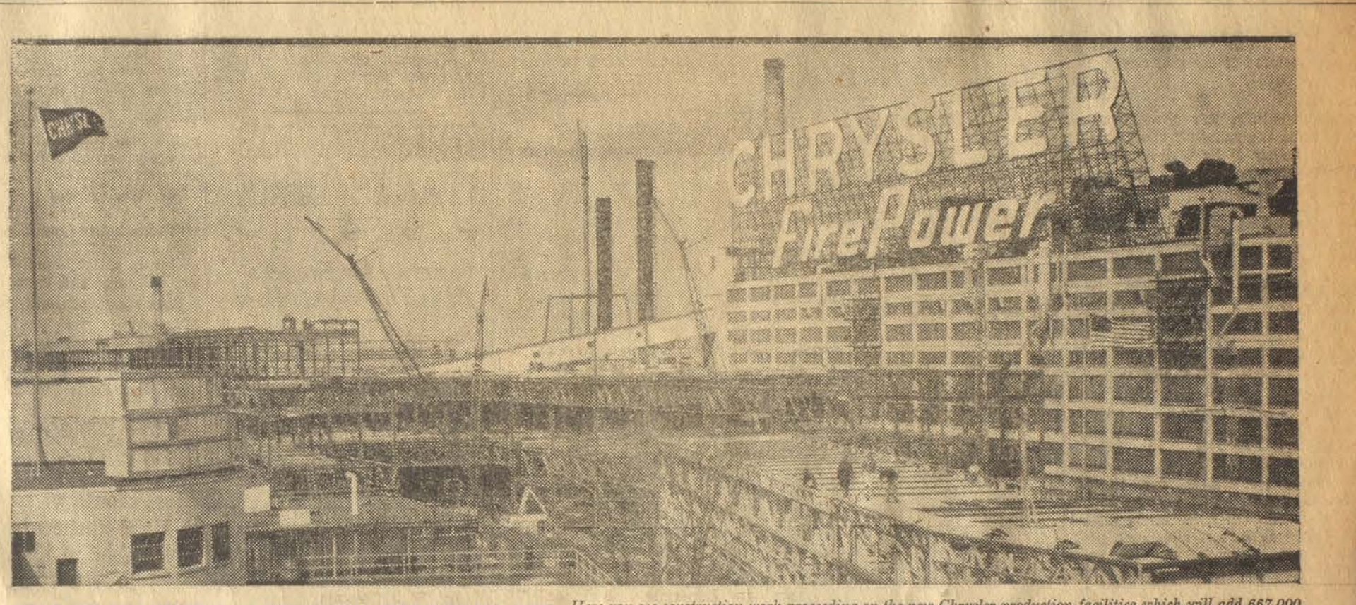
UP GOES CHRYSLER'S PRODUCTION MORE THAN 40% Here you see construction work proceeding on the new Chrysler production facilities which will add 667,000 square feet of floor space... including a 14-mile long continuous conveyor system, longest in the industry.
