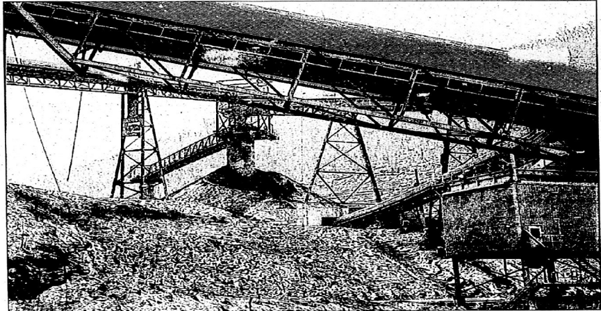
TECO, the parent company of Perry County Coal, announced last week the layoffs of around 90 people in Eastern Kentucky. Officials say six people were affected in Perry County. The above photo shows the conveyor lines at the Perry County Coal job at Boone Ledge.
