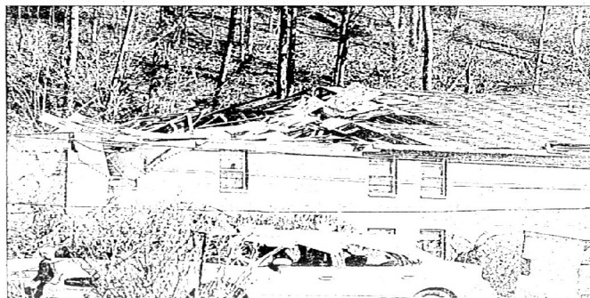
Several families at Pine Top Apartments lost their homes, after the tornado ripped the top off the building.
