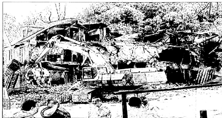
Work was underway Monday to demolish Wheelwright's old Clubhouse building. The building once housed a restaurant, a bowling alley and a barber shop, among other things. However, city leaders felt it was time to get rid of the structure and say a grocery store could go up in its place at some point in the future.
