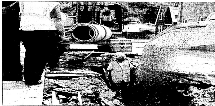
Utility workers were well underway with work along West Graham Street Tuesday morning as Prestonsburg officials continued the process of replacing the outdated and problematic sewer system currently in place. The overall project has a price tag of about $8 million.
