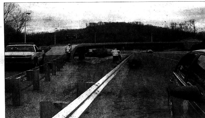
Work on the flyover bridge at Route 3 and Route 645 is nearly complete.
