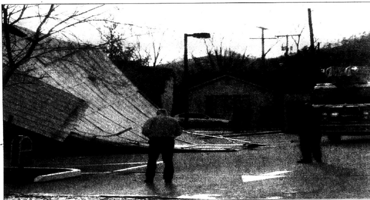
A strong gust of wind blew the roof off East Kentucky Physical Therapy in Prestonsburg on Wednesday. The high winds also downed trees and power lines in some parts of the county.
