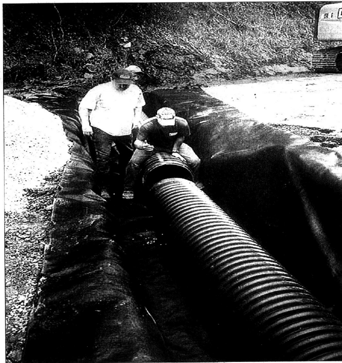
Highway Supt. Jerry Todd said the new cross drain on Route 40, between mile points 13 and 14 in Martin County, is made of plastic, a first for District 12. "The Transportation Cabinet just approved the use of these double wall plastic pipes for installation on state right of way," said. District 12 has a "plastic" walk bridge between River and Otter in Johnson County. Now the state highway department is using plastic drainpipes. "Plastic pipe has been around for a while," said Engineer Matt Moore, Section Supervisor for Martin County. "But it wasn't approved for use on state right of way until recently. The material won't rust, obviously, and it's much easier to install." Moore also said that plastic pipe is just as strong as its conventional metal counterparts. "It has to meet certain specifications as far as how much weight it will hold. What we used will hold just as much weight from vehicles as the metal drain pipes."
