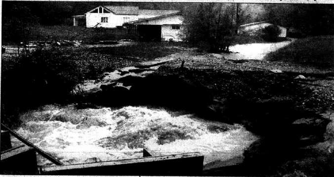
Heavy rains washed out a temporary culvert that had been built while a nearby bridge was being replaced, stranding several residents of Little Paint. The culvert was restored by Monday afternoon.
