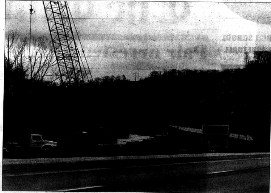
Route 645 flyover bridge looking from Inez side of highway east. You can see that there are two additional pillars that will be finished this year. photo by Sara George
