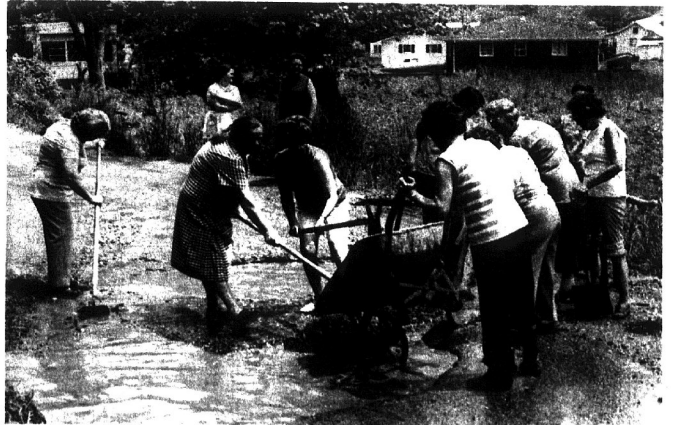
After repeated requests to the state highway department for road improvements had reportedly failed, this group of Dwale women decided last week to make certain improvements themselves—even without the use of road equipment. According to the women, the road, which is the approach to Dwale from new U.S. 23, has steadily deteriorated since the construction of new U.S. 23 a little over a year ago and caused serious drainage problems. The work involved ditching and draining the road and filling the ruts with rocks which they carried some distance.
