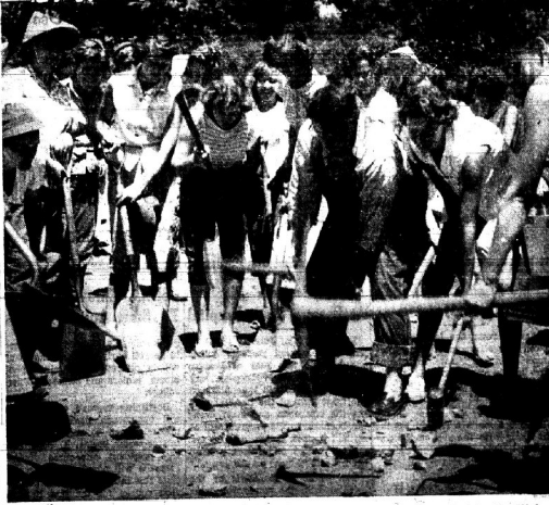
As women turn out to work recently on the highway in protest of its neglect by the Highway Department. The aroused women, besides wielding pick and shovel on the road, turned to with hammer and nails to repair the bridge over the Sandy there. Resumption of work on the road was promised by Rural Highway Commissioner J. B. Wells, Monday of this week.
