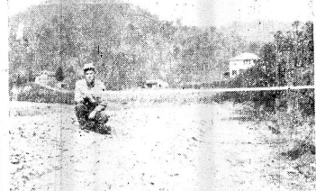
Duncan Rose, soil conservationist, with the Floyd county soil conservation district, showing width of open drainage work performed by John Allen and Forrest Burchett, of Sugar Leaf vicinity. It is 650 feet long and 10 feet wide. This conservation work added to the area of the field and provided for water run-off of Sugar Leaf Creek where none had existed.
