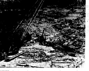
UNTIL LAST NOVEMBER the area where this dragline is working was a part of the Tennessee river bed at the TVA's Kentucky Dam site. One of the greatest of dams ever erected in dam construction engulfs the area, which covers about 60 acres. This giant dragline removes six cubic yards of material at a bite.
