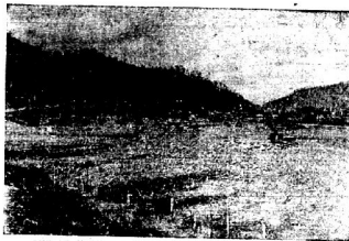
Mechanized might makes short work of filling level bottoms for the roadbed.
