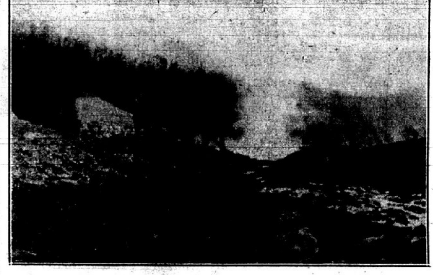
No longer a scene of rusticity is the head of Lick Fork of Middle Creek. Things are happening up there, as witness: Top photo: Looking downstream, top of tippie under construction in foreground. At left, machinery tearing away the mountainside for the railroad.
