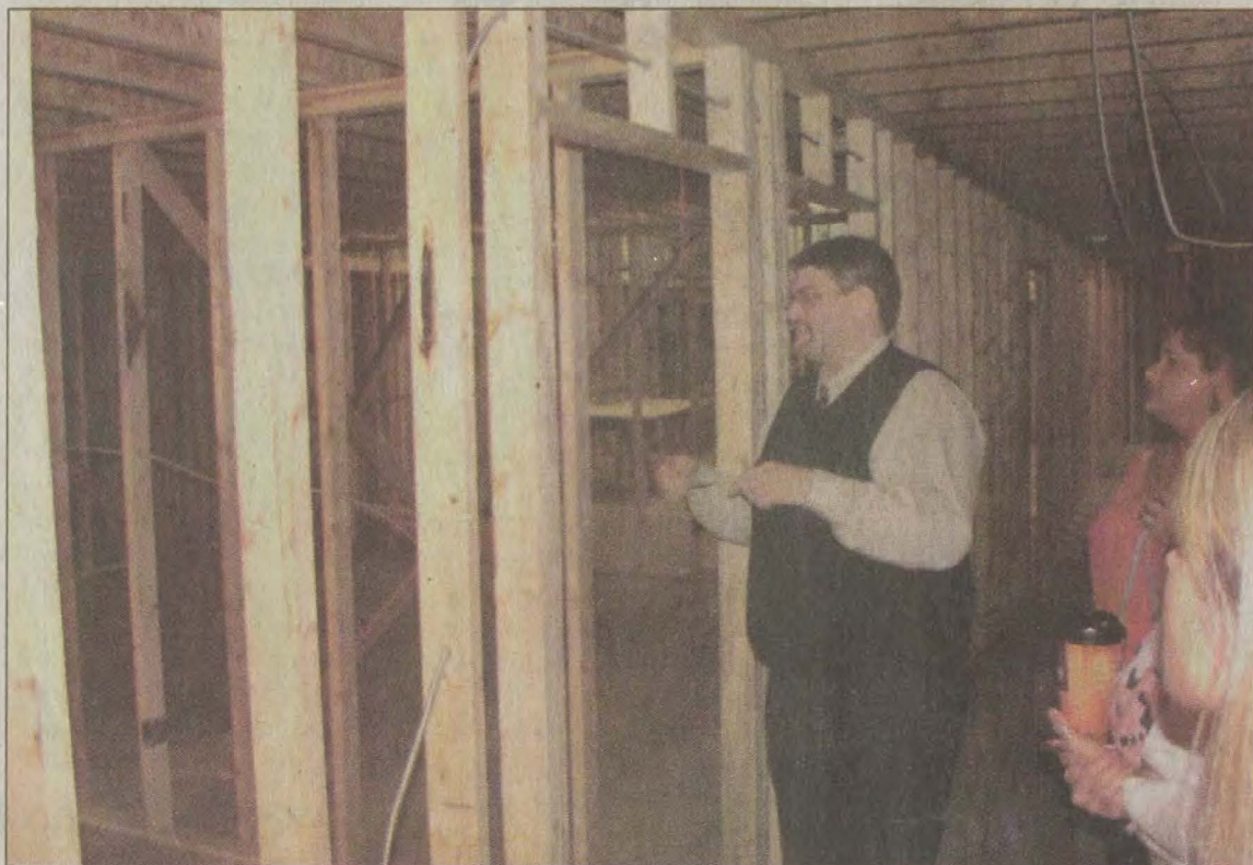
Thomas Rainey, director of the Carl D. Perkins Job Corps Center in Prestonsburg, leads a tour showcasing the construction work currently underway at the facility.
