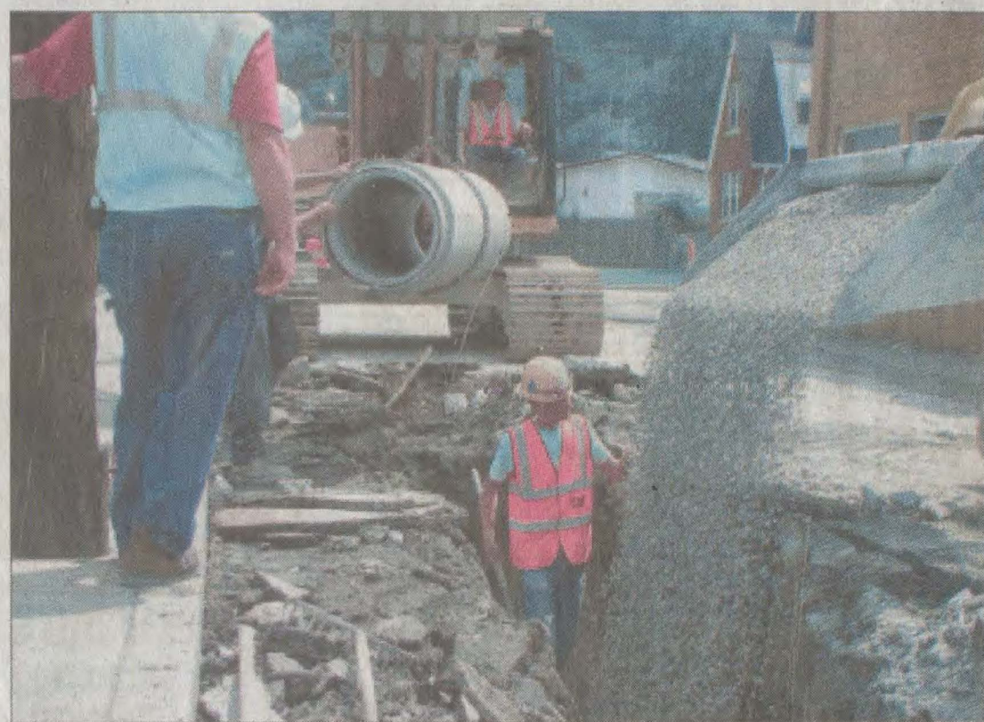
Utility workers were well underway with work along West Graham Street Tuesday morning as Prestonsburg officials continued the process of replacing the outdated and problematic sewer system currently in place. The overall project has a price tag of about $8 million.
