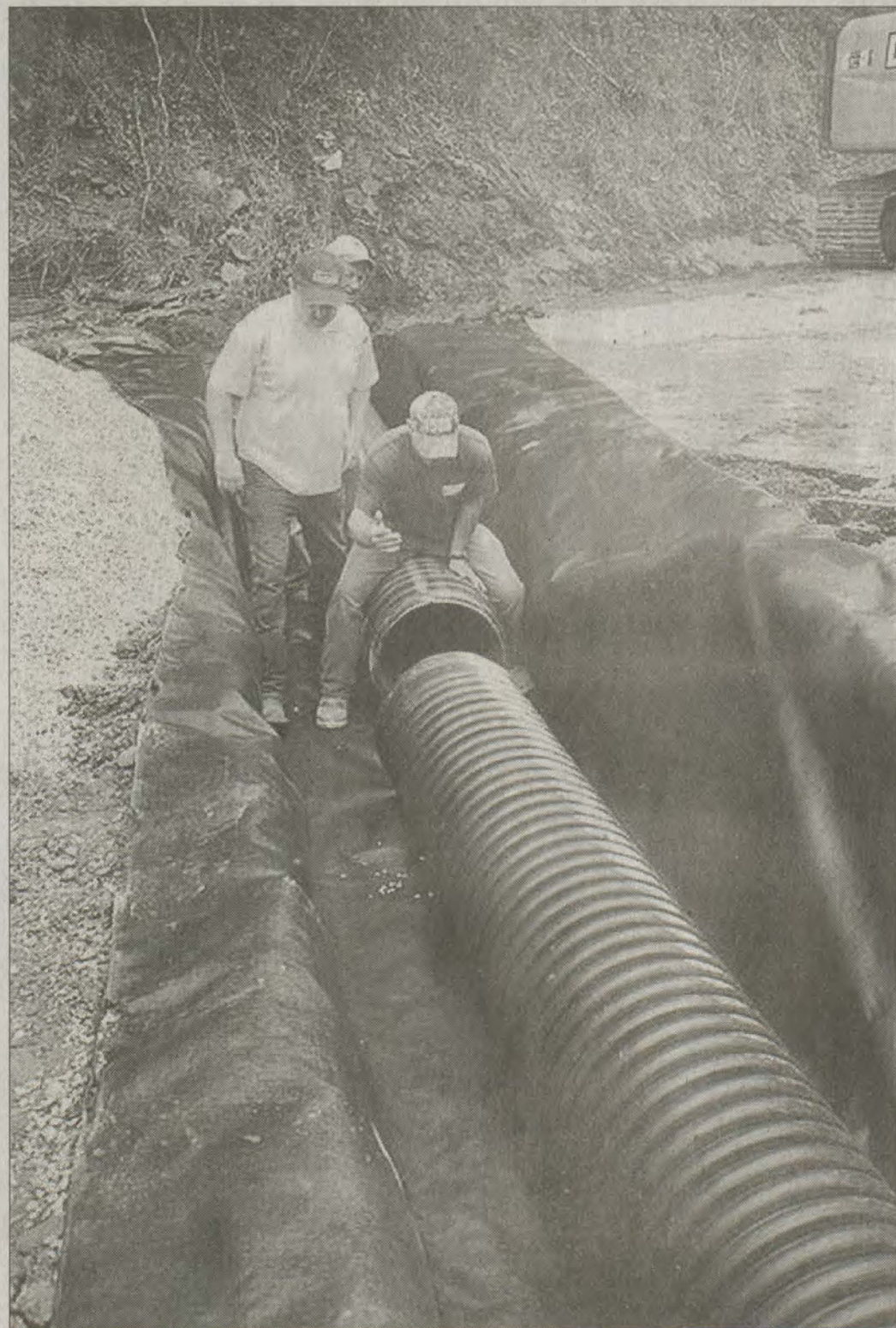
Highway Supt. Jerry Todd said the new cross drain on Route 40, between mile points 13 and 14 in Martin County, is made of plastic, a first for District 12. "The Transportation Cabinet just approved the use of these double wall plastic pipes for installation on state right of way," he said. District 12 has a "plastic" walk bridge between River and Offutt in Johnson County. Now the state highway department is using plastic drainpipes. "Plastic pipe has been around for a while," said Engineer Matt Moore, Section Supervisor for Martin County. "But it wasn't approved for use on state right of way until recently. The material won't rust, obviously, and it's much easier to install." Moore also said that plastic pipe is just as strong as its conventional metal counterparts. "It has to meet certain specifications as far as how much weight it will hold. What we used will hold just as much weight from vehicles as the metal drain pipes."
