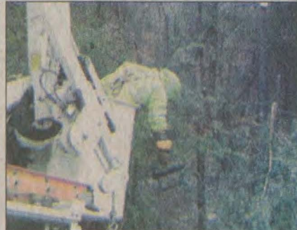
Electrical crews have been working around the clock to remove debris from power lines and restore electricity to thousands across the region. At left, an AEP worker toiled amidst fallen trees behind Jerry's in Prestonsburg.
