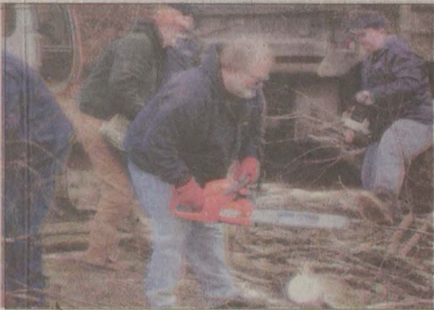
In the past week Floyd County District 1 Magistrate John Goble and crew members, along with crews from Districts 3 and 4, have worked 12 to 15 hours a day to clear fallen trees from roadways. Goble is pictured here with workers along Abbott Creek.
