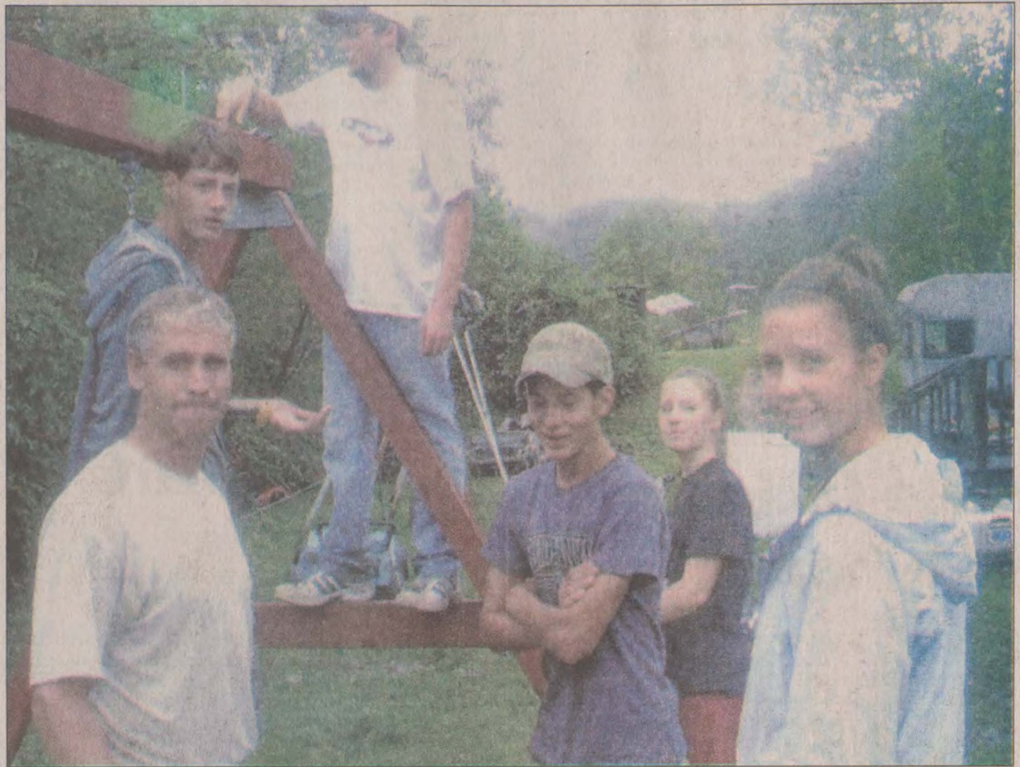
The Piarist School is playing host to 26 outreach workers from Wisconsin this week. The group is replacing and repairing windows at homes in Magoffin County until tomorrow.
