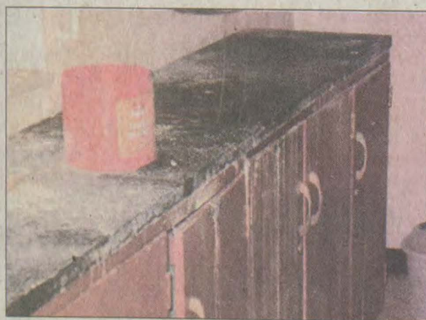
Water damage from the school's leaking roof is evident in this classroom.
