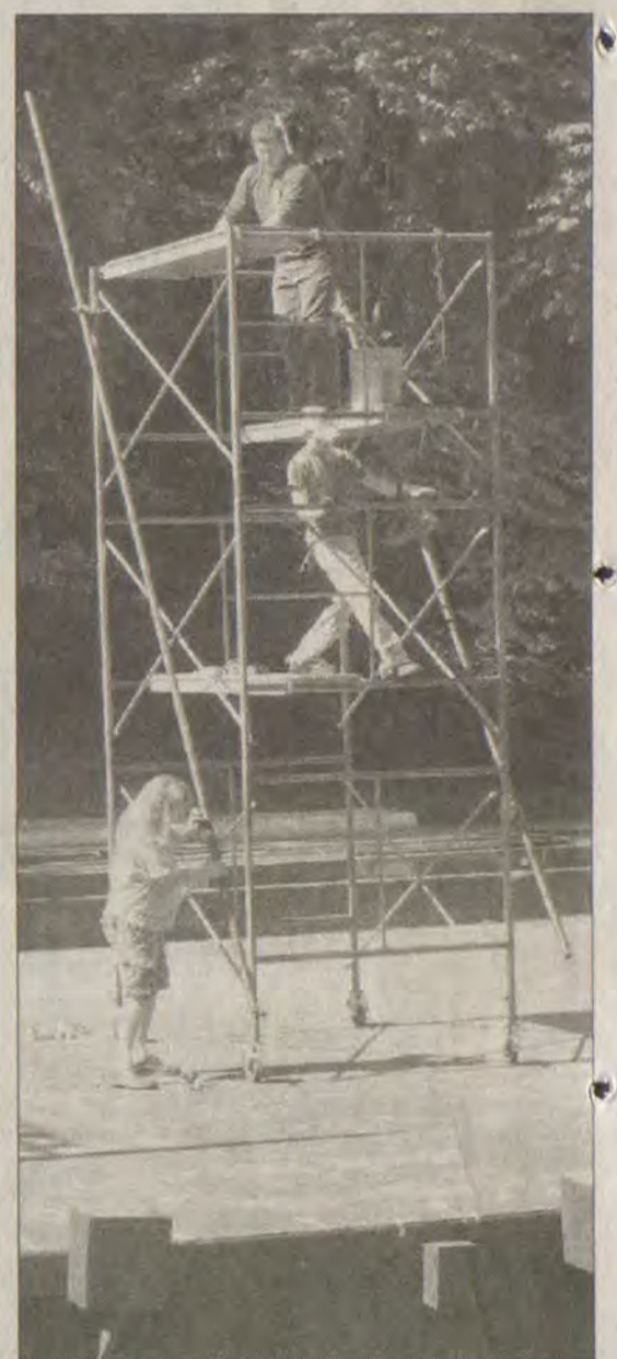
The Jenny Wiley Theatre technical crew begins the processing of repositioning and assembling the truss on which the new proscenium will be built.
