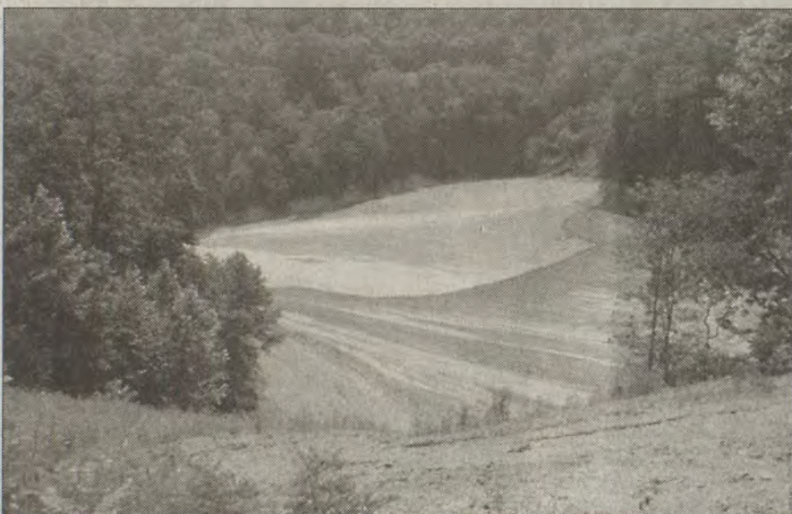
Cover placed over a low-permeable cap layer at the old Floyd County Landfill.
