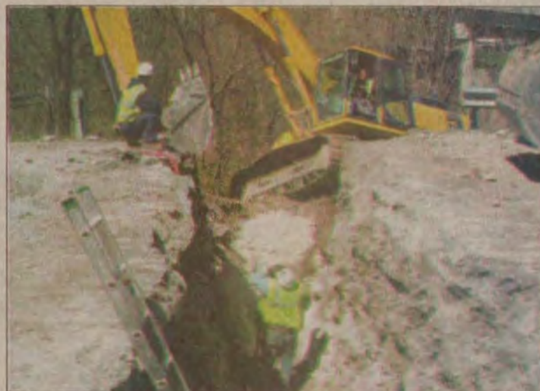
Mike Hatfield, Larry Riff and Curt Thomas worked this week to dig a trench for a new sewer line in Martin. The new line will connect to the city's new downtown area, as part of the Martin Redevelopment Project.
