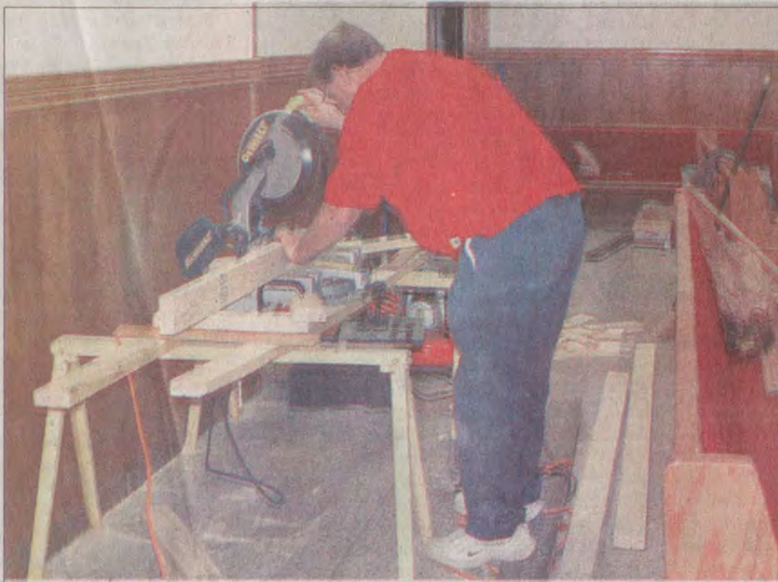
Workers were busy with remodeling the Floyd County Fiscal Courtroom Monday morning. Crew members expect to finish the project by Monday.
