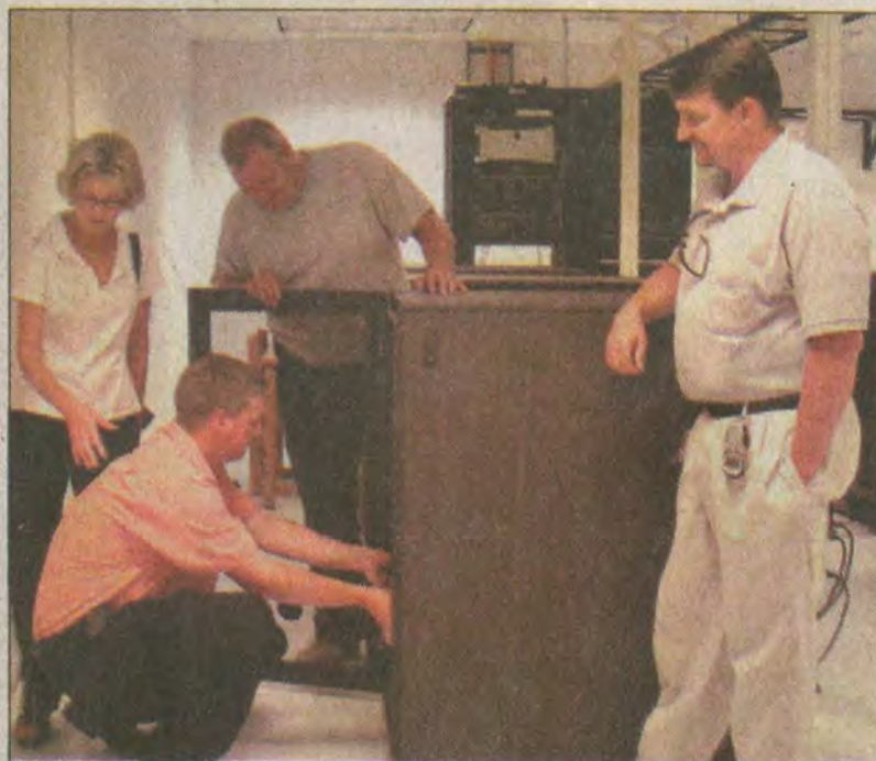
Network administrator Desmond Spencer explained the workings of the school district's new fiber-optic upgrade. This "hub" station at Prestonsburg High School connects all county schools with high-speed communications technologies. Also pictured are, standing front, Matt Wireman, standing back, Roy Harlow with Gearheart Communications, and Beverly Crisman.
