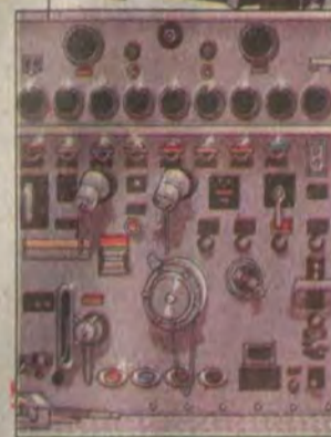
Pump control panel
