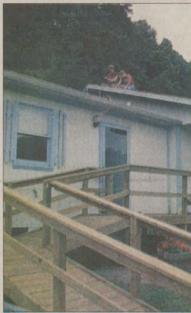
A work crew from the Auxier center built this ramp onto the home of Gary Michael and Linda Wright last week. This week, the crew is repairing damage to the roof of the couple's home.
