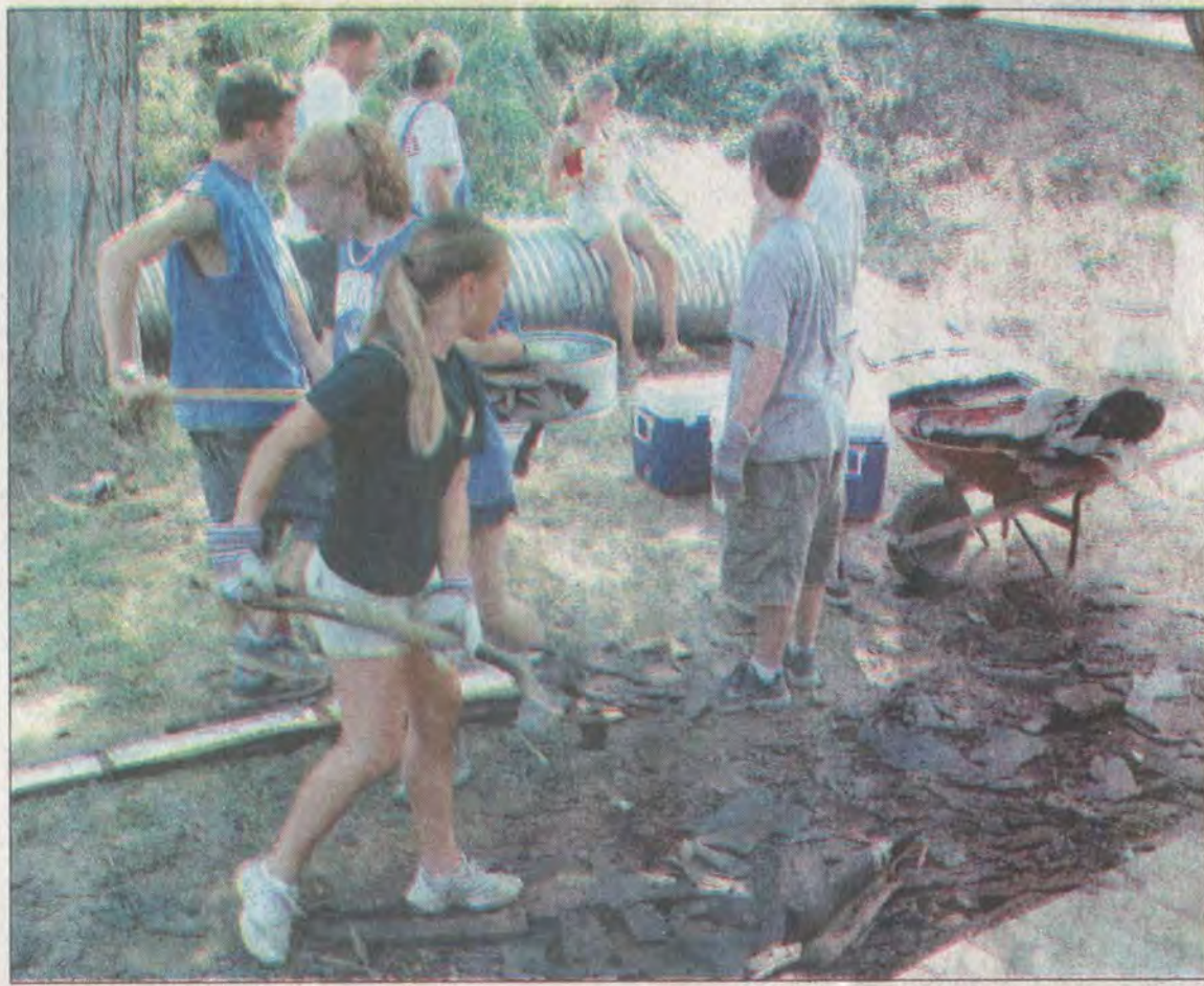
Volunteers from Connecticut spent their third summer vacation with LINKS this week and helped restore a home on Route 1750 that will be used to house LINKS workers when they visit the area to work for the organization.
