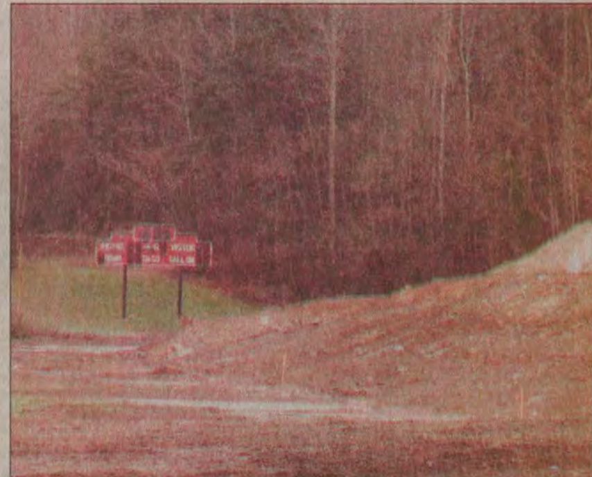
The football scoreboard is all that remains of the former Charles F. Clark Elementary School on Route 114. The school, which was demolished this year, will be replaced with a new building that will house students from Clark and Prestonsburg Elementary schools. Construction will continue next year on the new facility.
