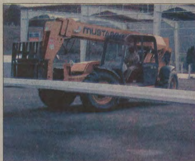
Construction of Layne Brothers Ford's 34,000 sq. ft. facility is continuing and is expected to be completed next year. Workers unloaded six truckloads of steel beams Tuesday for the "state of the art" facility. Fire destroyed the business, which has since relocated, and caused $4 million in losses in 2003.
