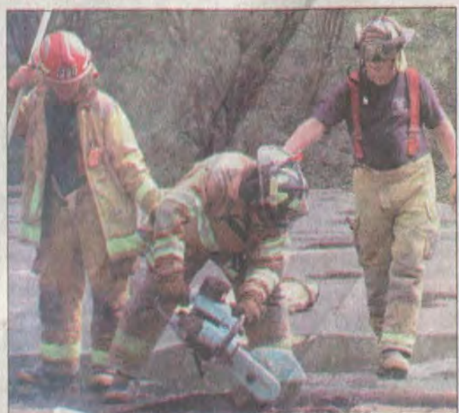
Firefighters used the K-12, a gas-powered circular saw, to cut ventilation holes and trenches in the roof at Clark Elementary. During a fire emergency, this practice helps ventilate smoke and gases from the building that could otherwise impede the rescue mission down below.
