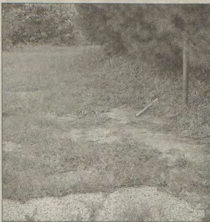
A few pieces of blacktop are all that remain of a 30-foot basketball court that was allegedly wrecked by a work crew installing a new sewer line for one Auxier resident.
