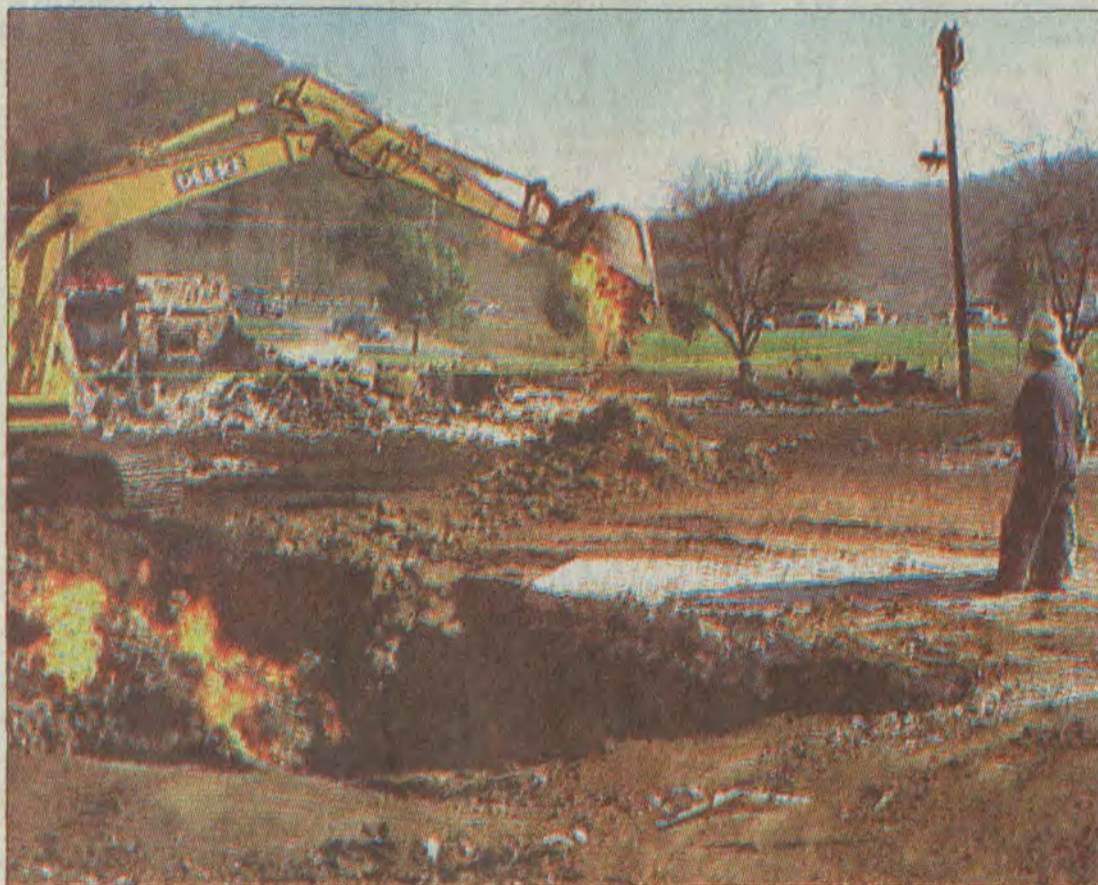
A backhoe was used to dig up the fractured section of pipeline. One of the odd facts about the fire is that the flaming debris is ice cold.
