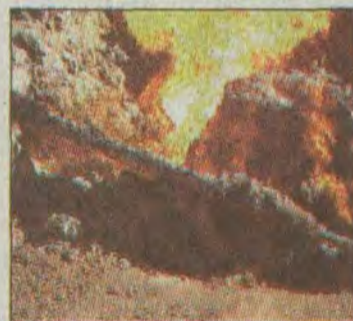
The broken section of pipeline from which the explosions emanated at Rolling Acres Monday is shown here after being unearthed by excavation workers.
