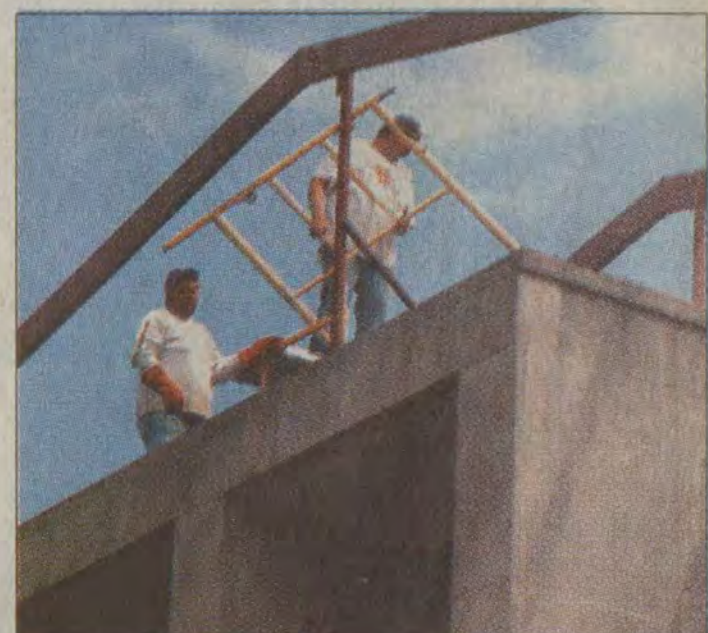
Work began last week to fix the roof of the Floyd County Courthouse.
