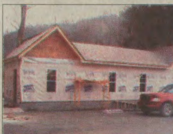
Construction is just about finished on new kennels for East Kentucky Rescue. The new climate-controlled building will house dogs awaiting adoption at the Stanville home of Lisa Scalf.
