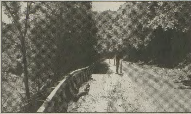
Crews inspected damage on Route 292 in Martin County, a state-maintained road that runs roughly parallel to the Tug Fork of the Big Sandy River from Pike County through Martin County.
