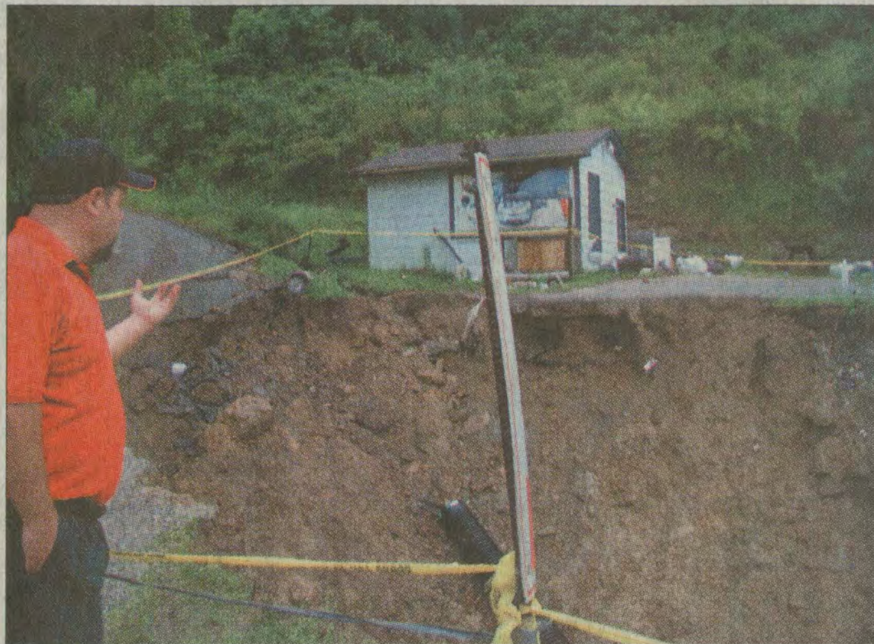
Fred Spears overlooks this gaping hole currently obstructing the Steel House Branch road on Route 302, which apparently occurred when a culvert washed out during Memorial Day flooding.
