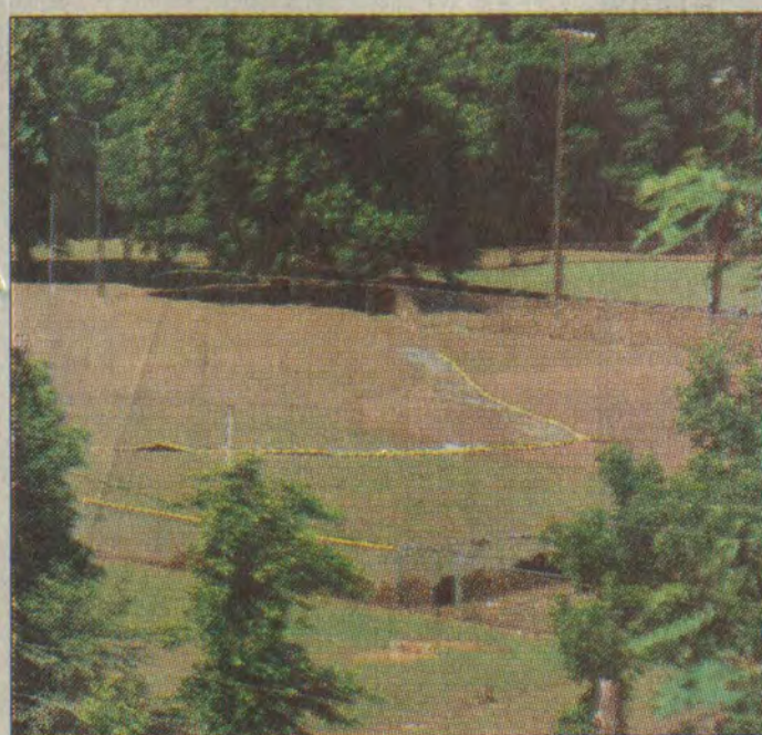
The fence at the Archer Park Little League field was uprooted following heavy rain.
